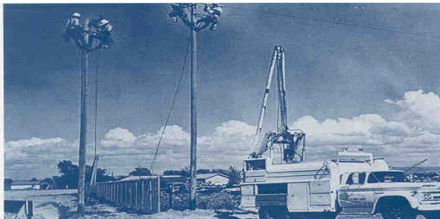
During the 1960s, crews worked hard to meet the increased demand of power needs.
